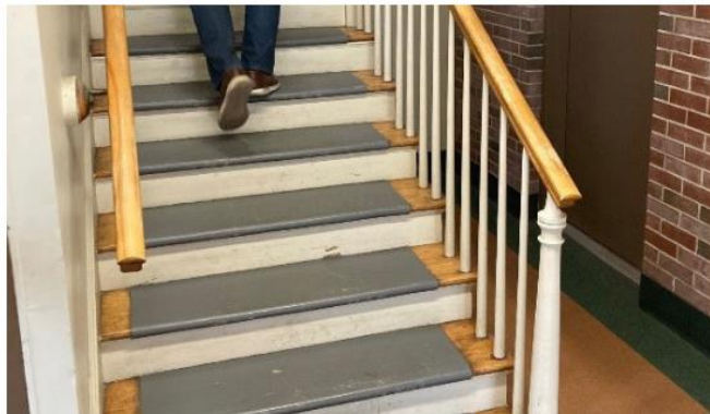
Inaccessible stairs lack code compliance.
