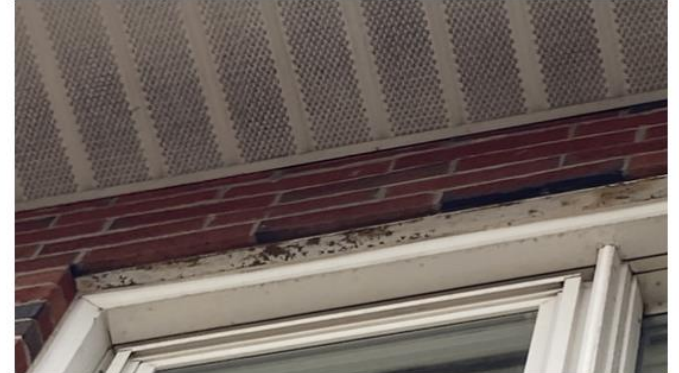
Rusted lintels and displaced bricks.
