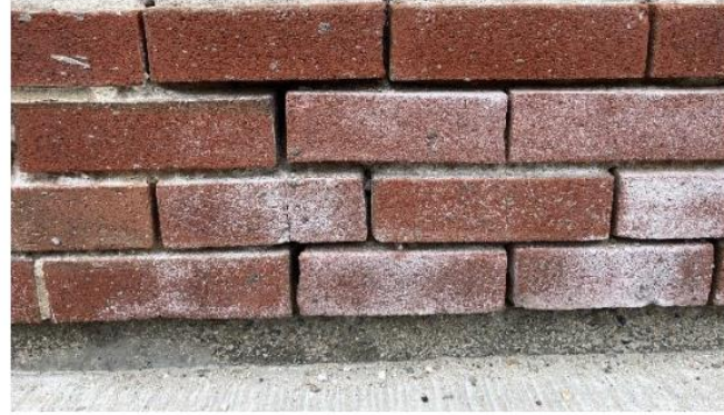
Degraded mortar and brick misalignment.
