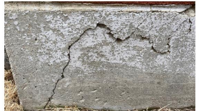
Cracking foundations and uneven settlement.
