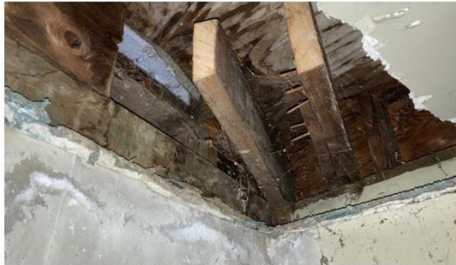
Floor framing rot and water damage.
