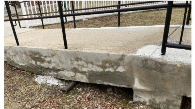
Damaged ramp with repeated failing repairs.
